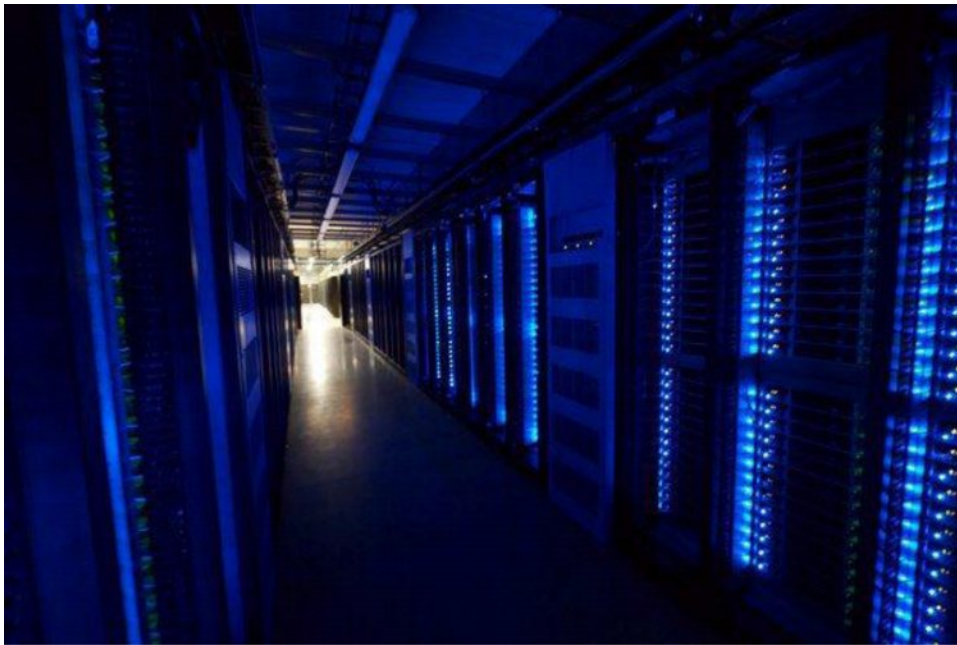
FIGURE 11.9 Facebook data center aisle.
