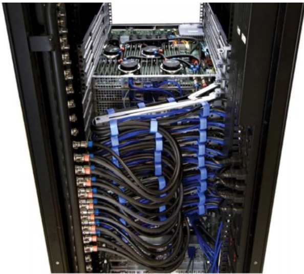
FIGURE 26.10 Water pipes and manifolds. Courtesy of Asetek.
