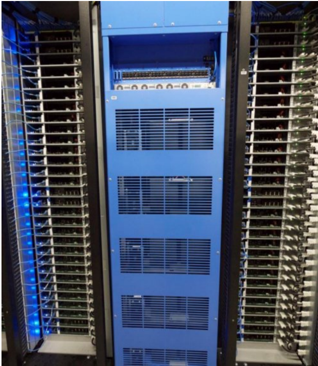
FIGURE 11.10 Facebook DC UPS battery cabinet.
