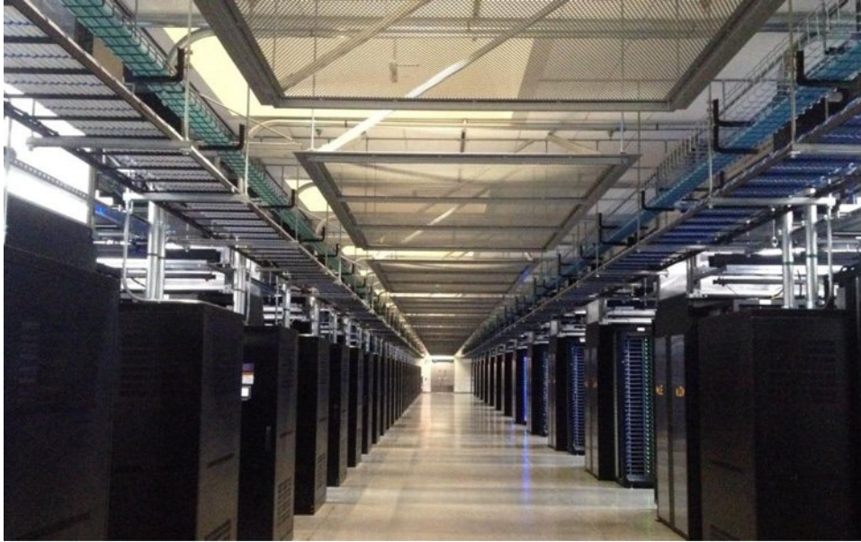
FIGURE 11.8 Facebook data center suite.
